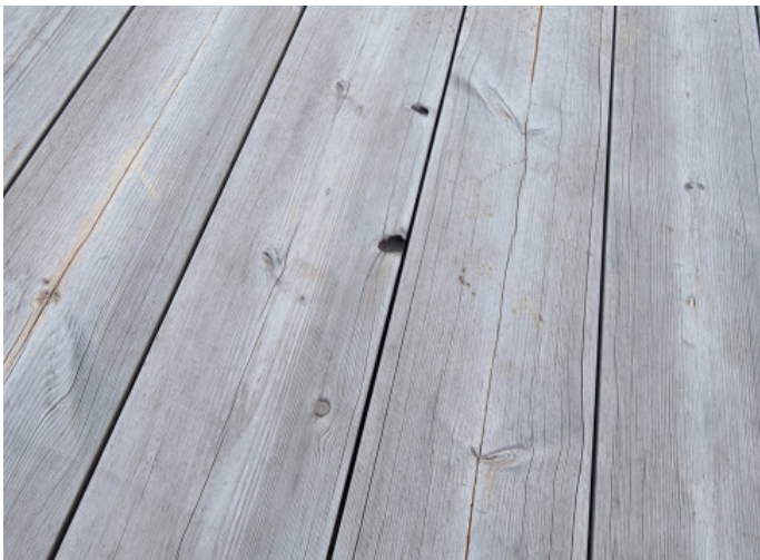
Untreated Lunawood decking 2 years after installation. Small hairline cracks can be seen on the surface.
