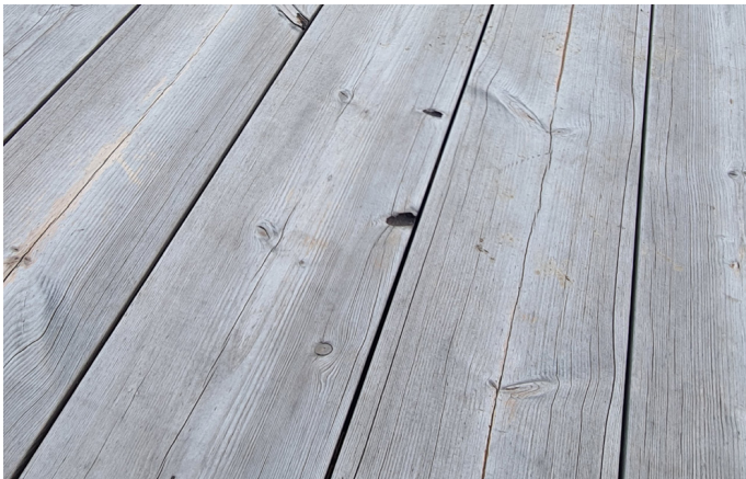
Untreated Lunawood decking 2 years after installation. Fine hairline cracks can be seen on the surface.
