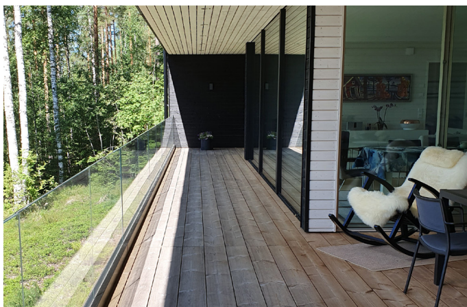
Lunawood decking 2 years after installation. The decking in the sunny area has turned gray faster compared to the shaded area.
